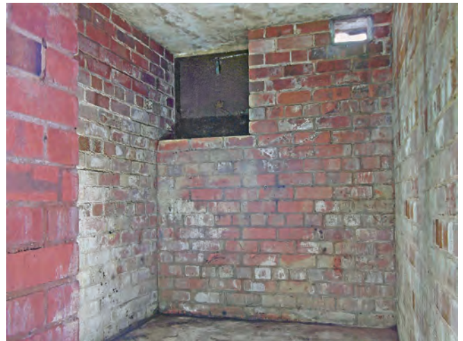
Emergency escape hatch in the second shelter
